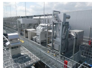
VOC Combustion Removal System
