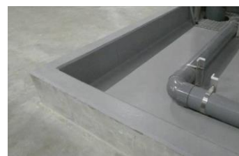
Dike (Waste Water Relay Tank)
