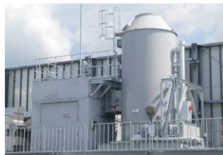
System for Cleaning Exhaust Gas
