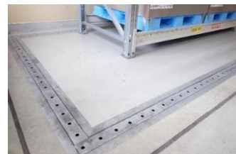
Prevent Leakage Pit
