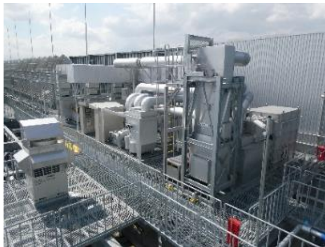
VOC removal system
